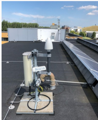
Figure 1: GPS/Galileo and DCF77 antennas on SIDN's roof
